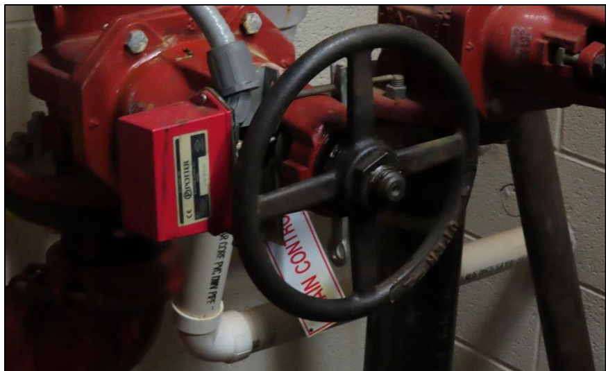
Figure 3.F Adair RJDC Sprinkler Shut-Off Valve And Labeled Handle
